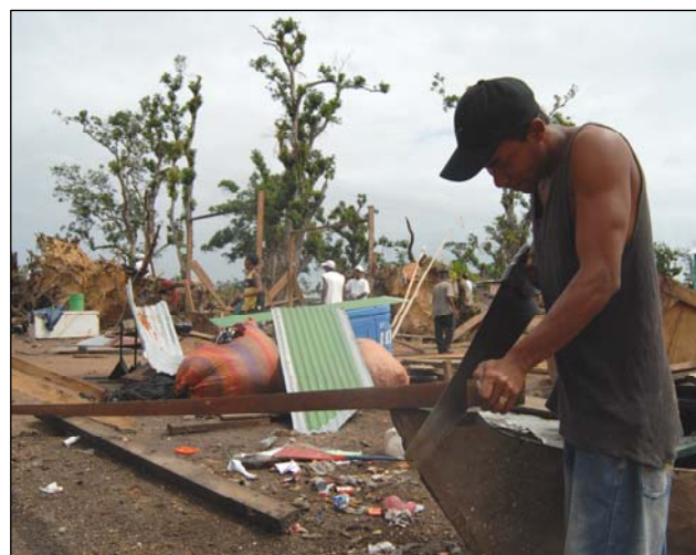
Krukira Region, Nicaragua. A beneficiary from the Techo programme cutting wood to repair his roof. The wood used to repair the roofs comes from the trees fallen after the passage of Hurricane Felix. (Photo: UNV/Mario Rizzolio)
