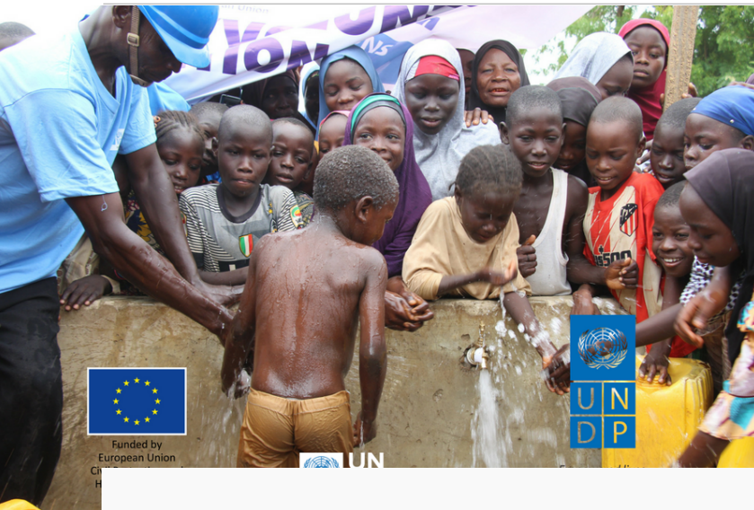
Children celebrating after successful repair of a borehole by UN Community Volunteers in Bara Community - Yobe State, Nigeria. @UNV 2018
