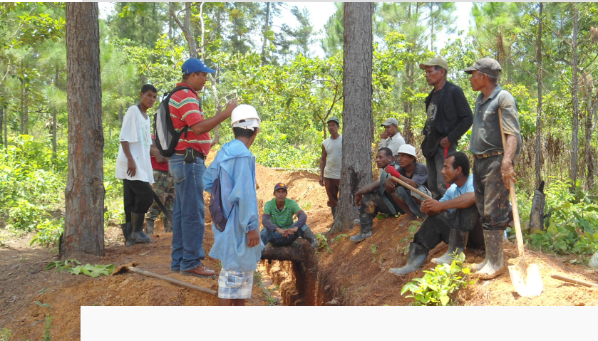
Meeting in Waspam, Nicaragua, among community members, the community leader, and the Committee for Potable Water and Sanitation during the installation of water pipes, assisted by the municipal engineer from Uhri. (UNV Program, 2012)
