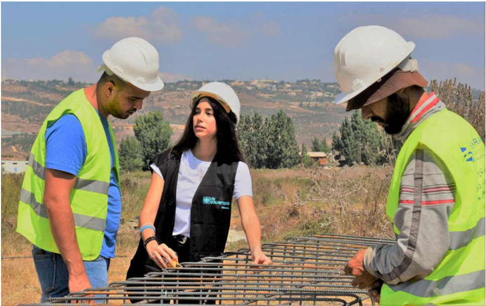
UN Youth Volunteer Zeinab Chamas monitoring work on upgrading irrigation infrastructure in South Lebanon. © UNDP, 2019
