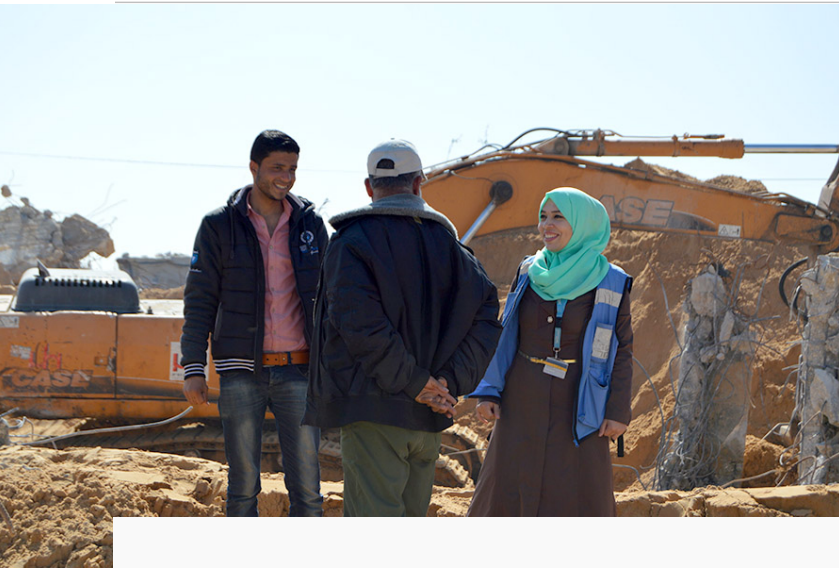
Mona Ouda, UN Volunteer engineer, supervising the removal of rubble for the rebuilding of schools in the Gaza Strip, State of Palestine. (UNV, 2016)
