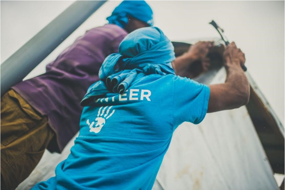
An All Hands volunteer and local Fijian rebuilding a home in Delakado village in Fiji (2016). © All Hands Volunteers
