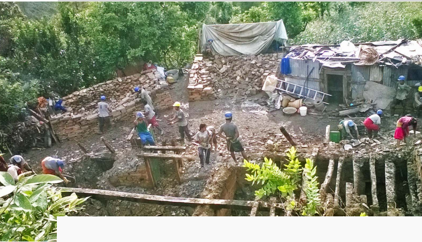
Volunteers working in the UNDP Demolition and Debris Management Project in Nepal in 2015.
