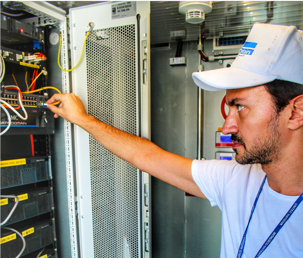
UN Volunteer David Bzhania making sure that the servers of the modular data center located in Goma, DRC are up and running. (Fairve, UNV, 2016).
