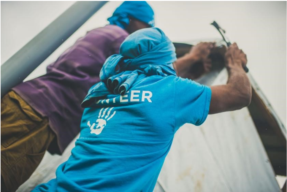
An All Hands volunteer and local Fijian rebuilding a home in Delakado village in Fiji (2016).
